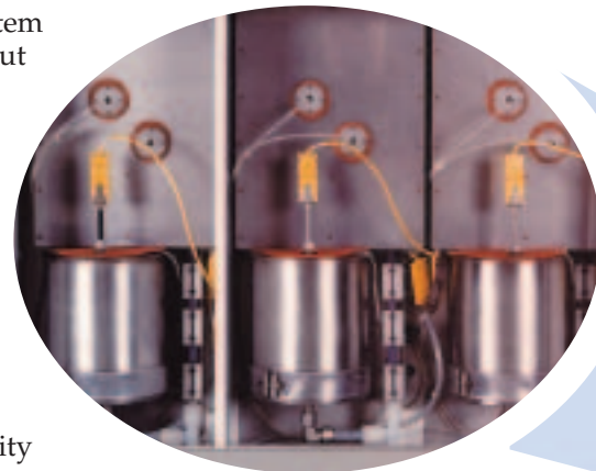
Level and temperature controlled chemical vapor bubblers
