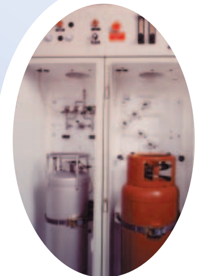
Bulk chemical storage and refill system
